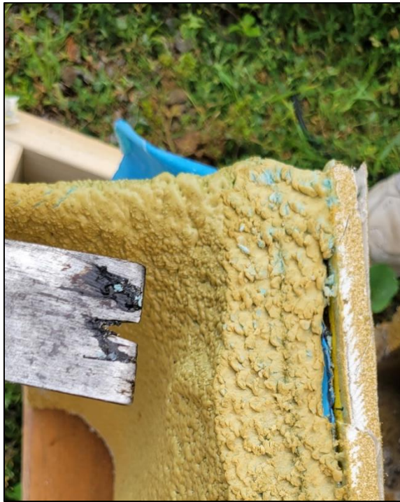
Figure 8. First attempt to remove SealTite One from exterior glass faced gypsum. Prybar shows bitumen intact.
