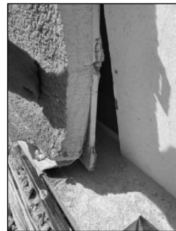
Figure 1. Shrinking foam causing Blueskin TWF to peel from exterior glass faced gypsum.
